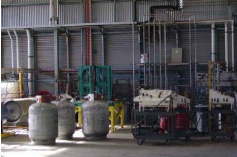
Containers should not be stored in confined spaces.
