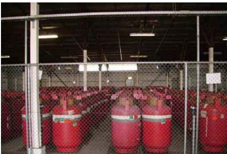
Storage areas should have good physical security to protect against hazards and theft.
